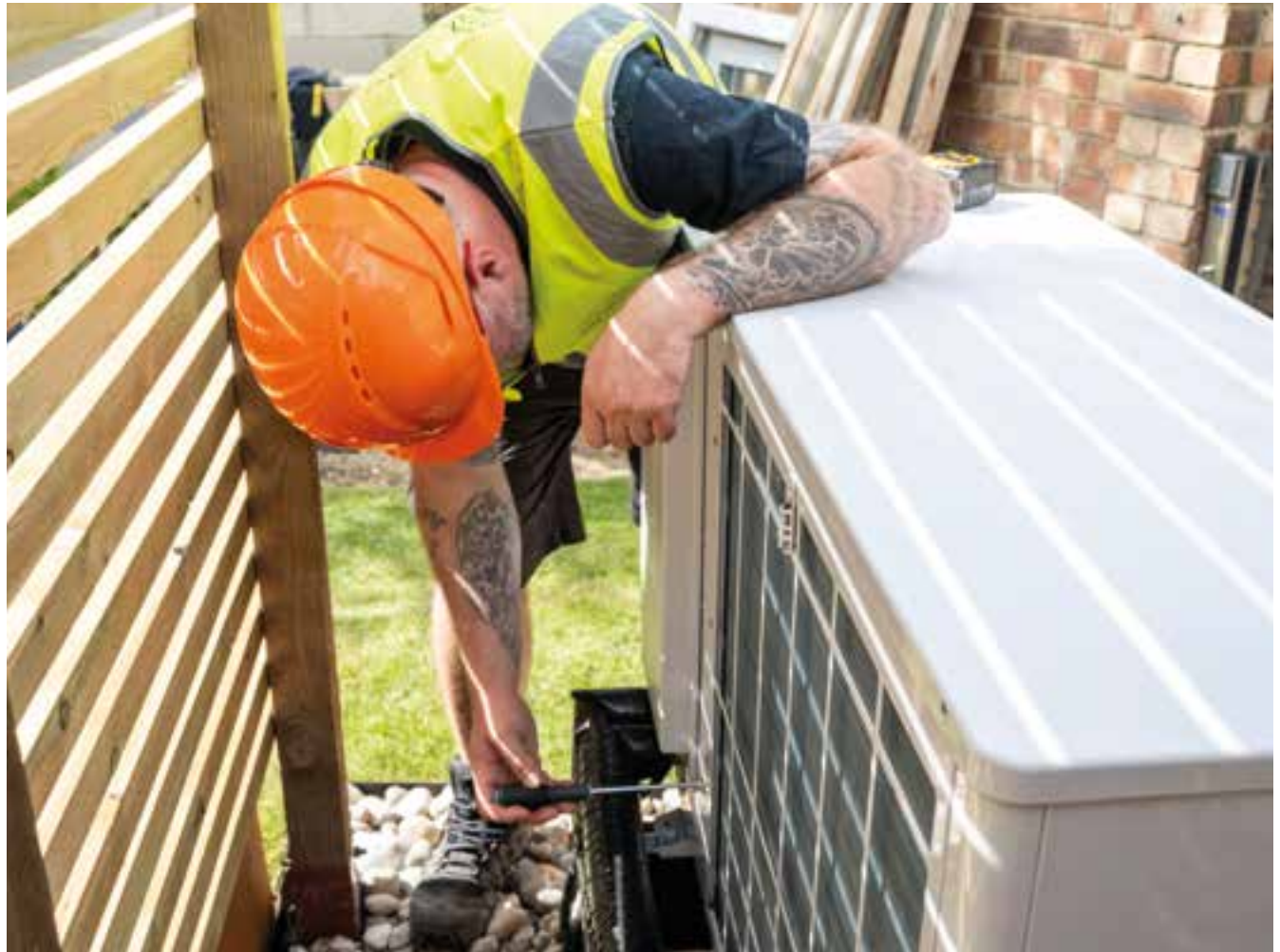
Image: Maintenance of a residential ground source heat pump.
